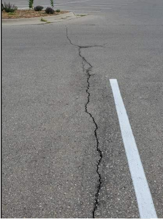
Cracks in the South end of Main Lot
