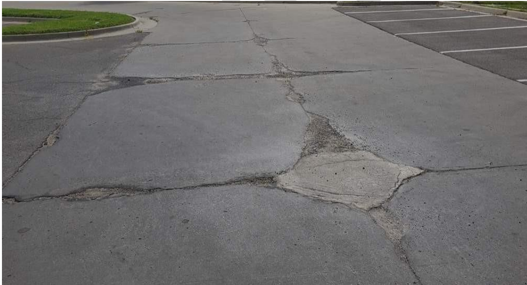
Damaged Concrete Drive Aisle – East side of the main lot
