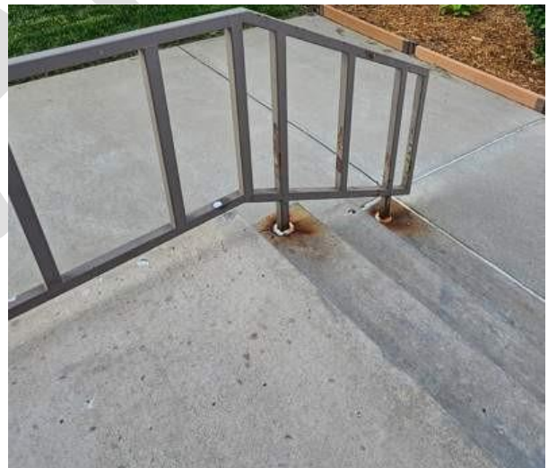
Chipped paint and rust development.
