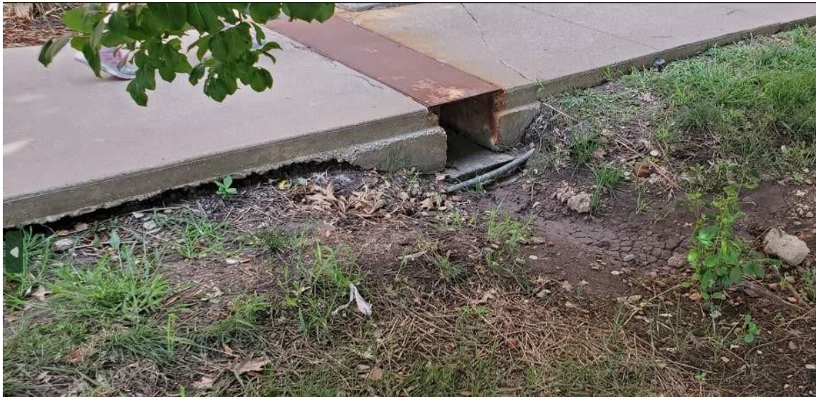
The north sidewalk along 10 th Ave. where frequent discharge from the Overflow drain is cutting out the embankment.
