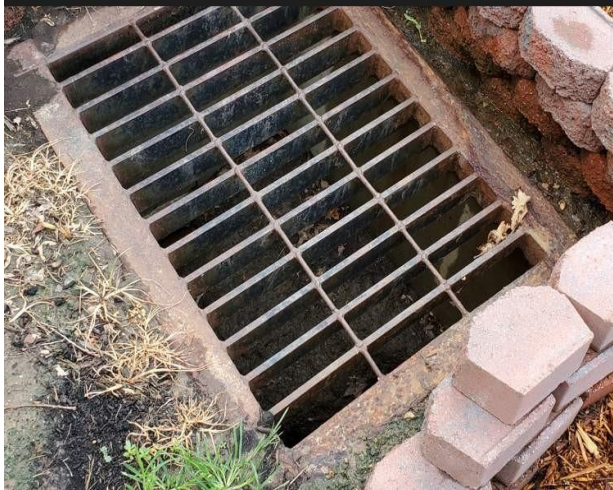
SE Corner Inlet containing dirt and mulch.
