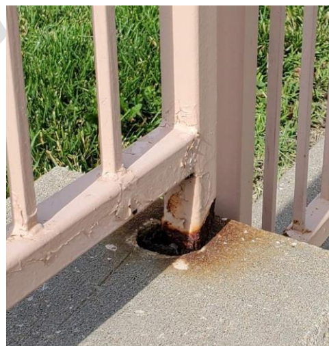
Rusted through vertical – Loading Dock wall.
