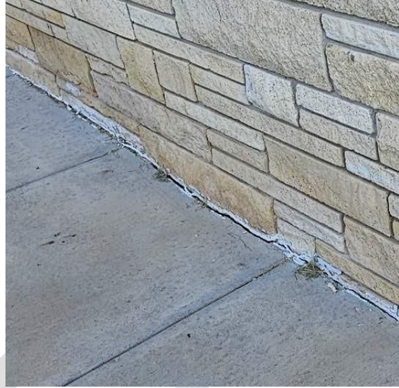
Sealant joint failure between wall and sidewalk.
