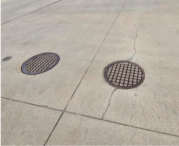
Crack at Sand/Oil Separator – East Side
