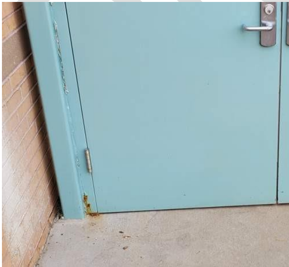
Rust and Sealant Failure – Amphitheater
