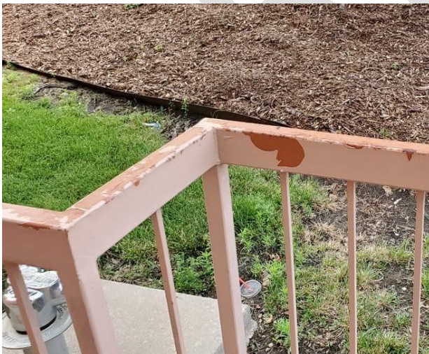
Flaking paint on rails and verticals
