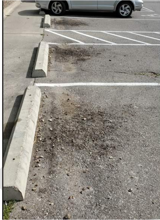
Rutting at Accessible stalls – Main Lot
