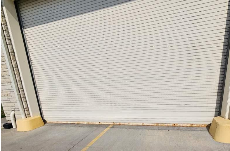
Rust starting on bottom angles of coiling doors.
