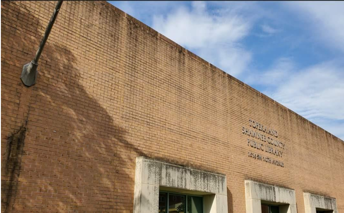
Various examples of masonry staining.
