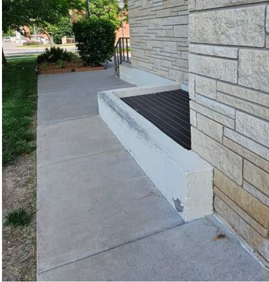
Grind marks on the concrete wall's upper edge.
