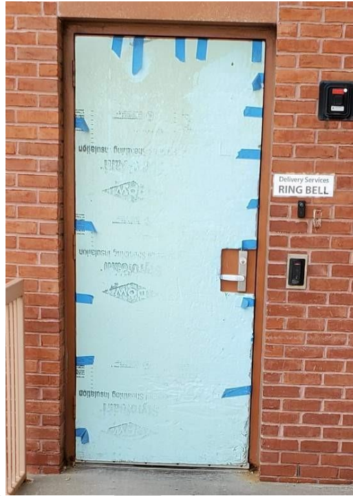
Possible uninsulated door.
