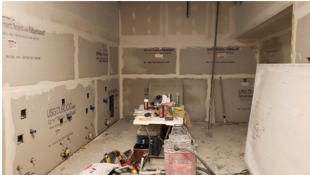
Restroom near café with cement board installed in preparation of new tile
