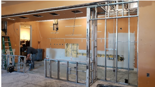
Millennium Café with framing for new counter and grab and go cooler niche
